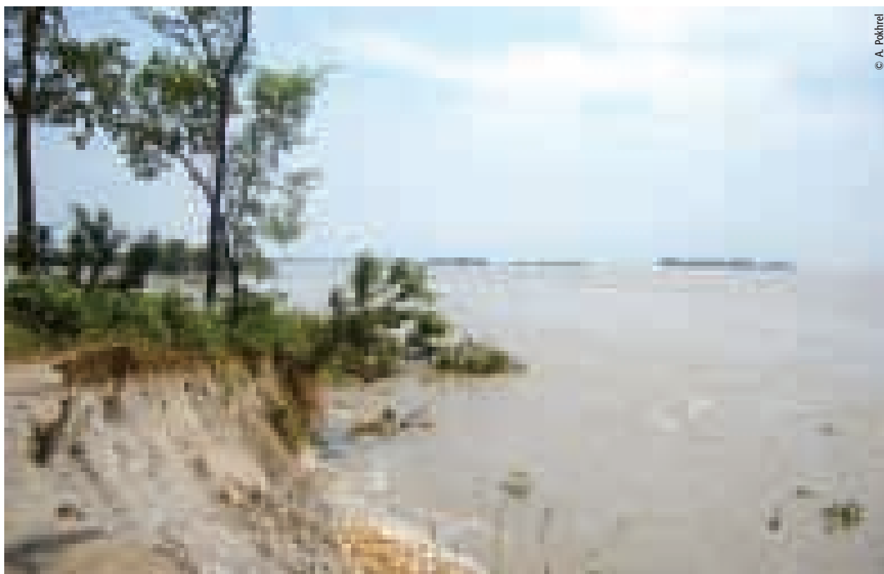
FIGURE 5 | August 18, 2008 Kosi embankment breach site at Paschim Kusaha, Nepal
