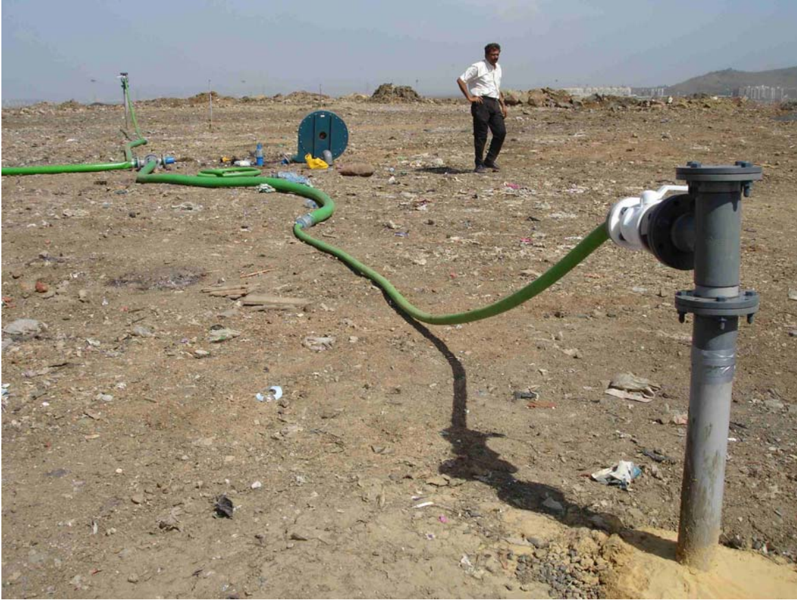
Figure 3-5. Pump Test Extraction Well, Blower, and Collection Piping
