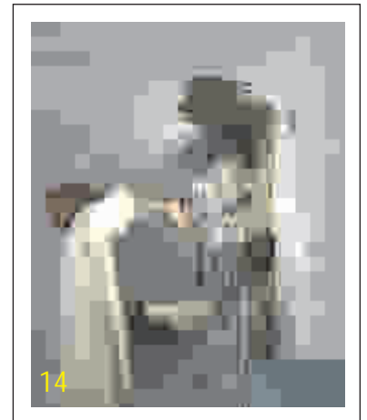
14. Wet the slab and apply neat cement slurry followed by cement mortar in 1:3. Finish it to match surrounding area. Cure for 15 days.
