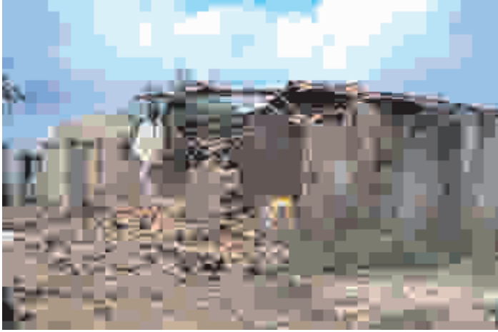
Collapse of wall and damage to roof
