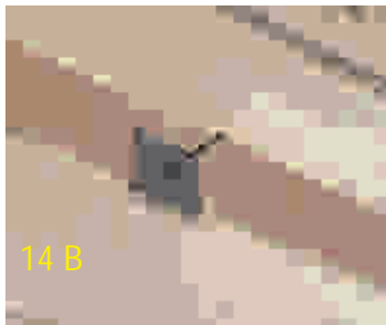
14.B Tighten the Tie rod, after finishing the belt, with the help of two nuts at each end. Place 75x75x5mm bearing plate in front of the nut before tightening.
