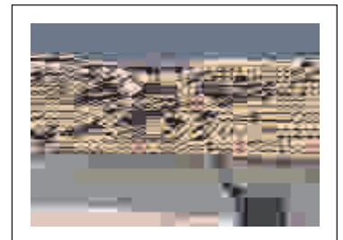
Roof distortion damage
