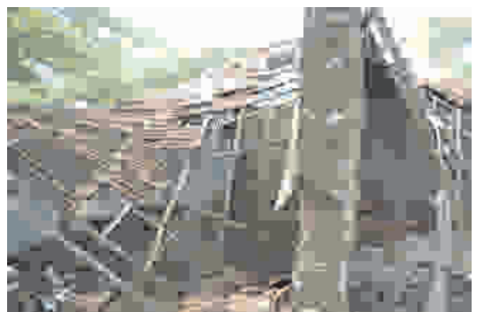
Wall & Roof damage by Cyclone
