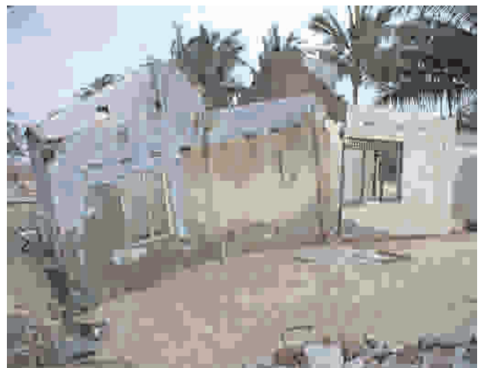
Damage due to foundation settlement
