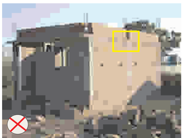
Never construct RCC columns without constructing beams resting on it and fully connected to it.
