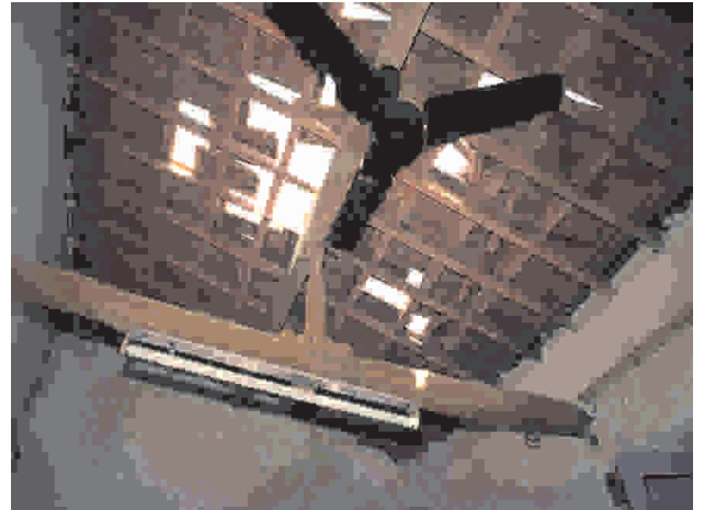
Roof Tiles blown off
