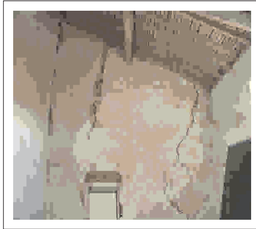
Moderate and fine cracks
