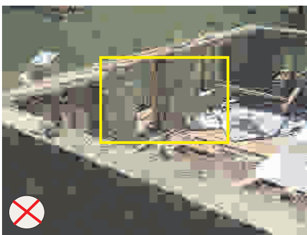
Never construct outside walls without constructing interior walls at the same time and fully connected to them.
