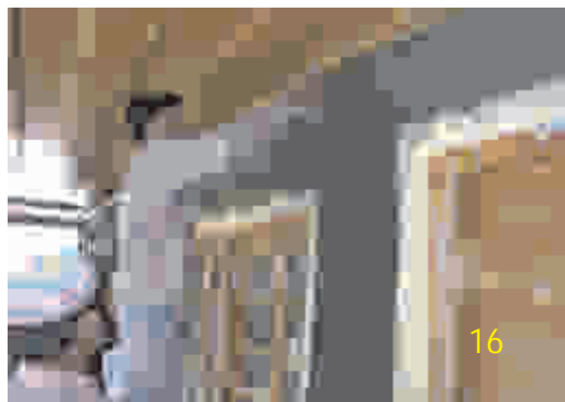
16. Place plaster in two coats, each 12mm (1/2") thick at an interval of 1 to 2 hours to provide 16mm (5/8") cover over the reinforcement.
