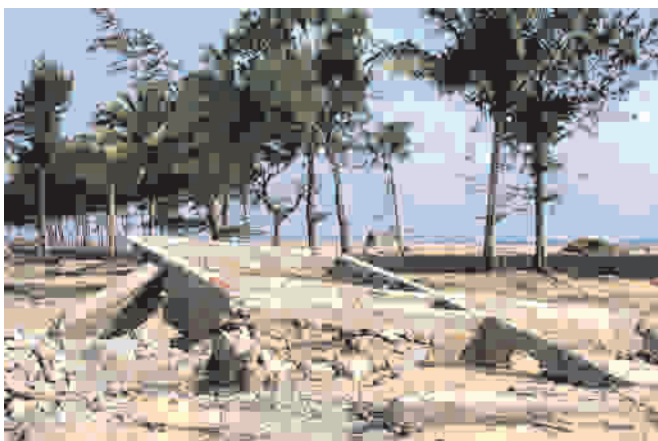
Damage by Cyclonic Surge
