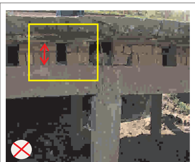
Never build RC slab without full connection with the beam.
