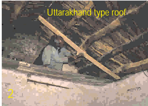
2. Using two nails at each end install a 100mm (4") x 25mm (1") strut (plank) on the underside of purlins adjacent to their ends.
