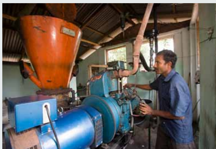
Adding woodchips to gasifier to produce energy
