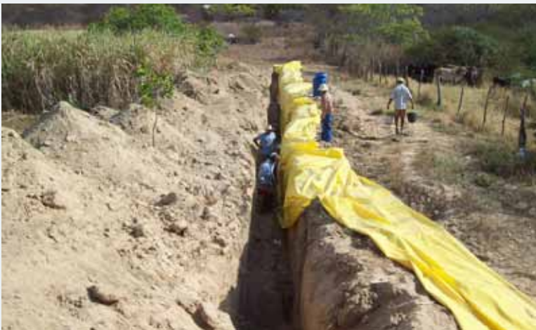
A tarpaulin is placed against one of the sides of the trench and fixed at the bottom with concrete. The trench is then filled in again. The rain water seeping into the soil is prevented from seeping downhill, creating a marsh.
