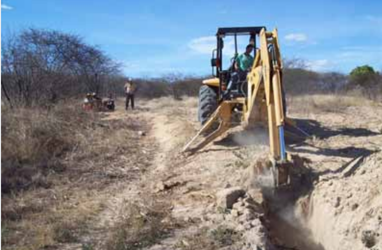
Digging trench – the first step in underground dam construction (Here they are lucky to have a digger and hence don't have to dig with shovels and picks)
