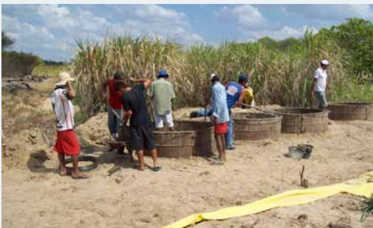
Making concrete rings for lining wells and water tanks. On the side of the marsh, wells are dug and lined with concrete rings, which fill up with the water less the soil.
