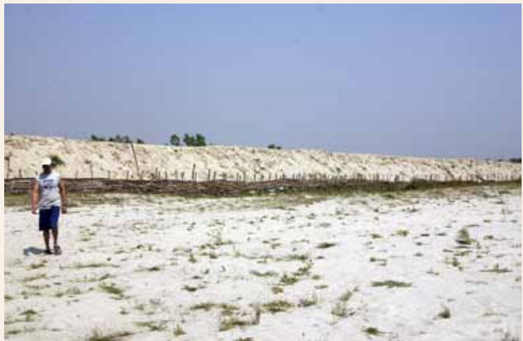
River embankment, using bioengineering in eastern Nepal, working area of LWF Nepal. ©LWF Nepal
