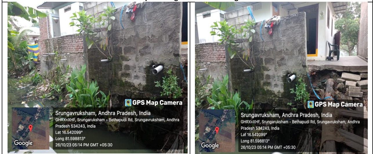
Sewage and Toilet pipe line outlets of Srungavruksham Grampanchayat are connected to Irrigation Pipe No.10 (agricultural filed bhodhi)
