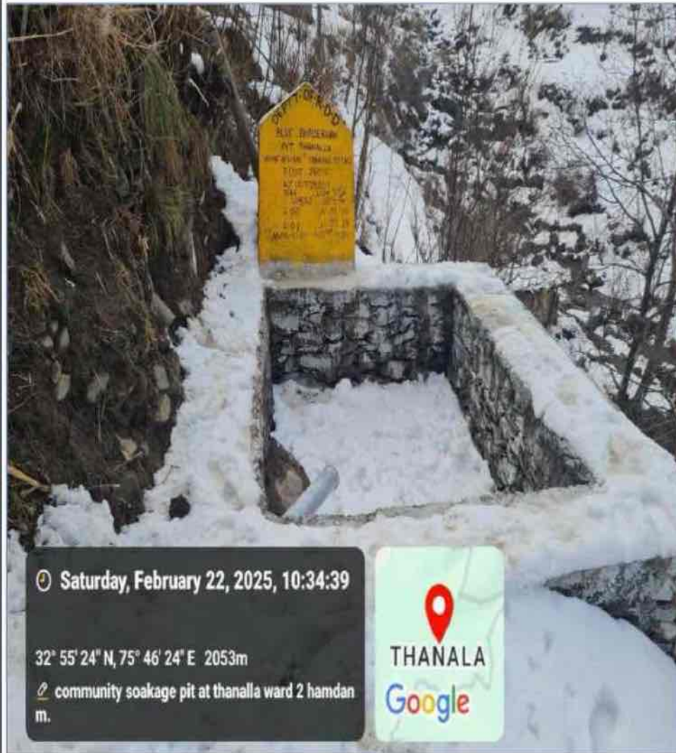
COMMUNITY SOAKAGE PIT AT THANALLA
