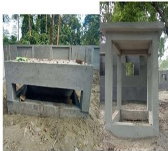
DG Pad and Transformer Shed
