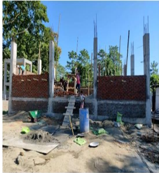
Sludge Storage shed and Over Head Tank
