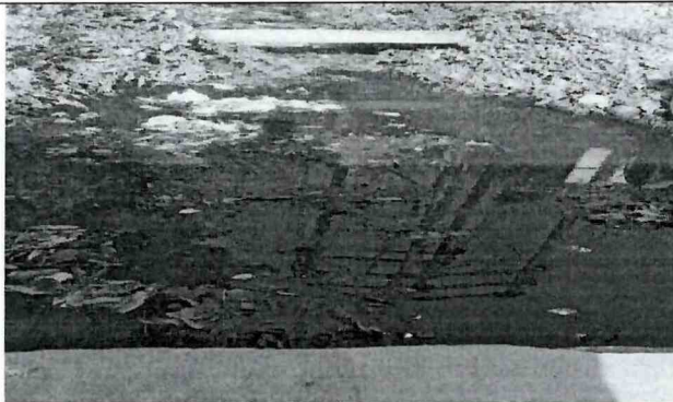
Fig:3 Presence of wastewater in the storm water drain
