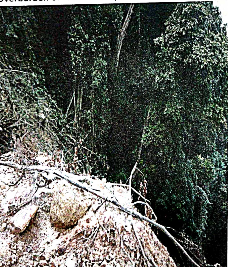
Overburden of rock & soil spillage:
