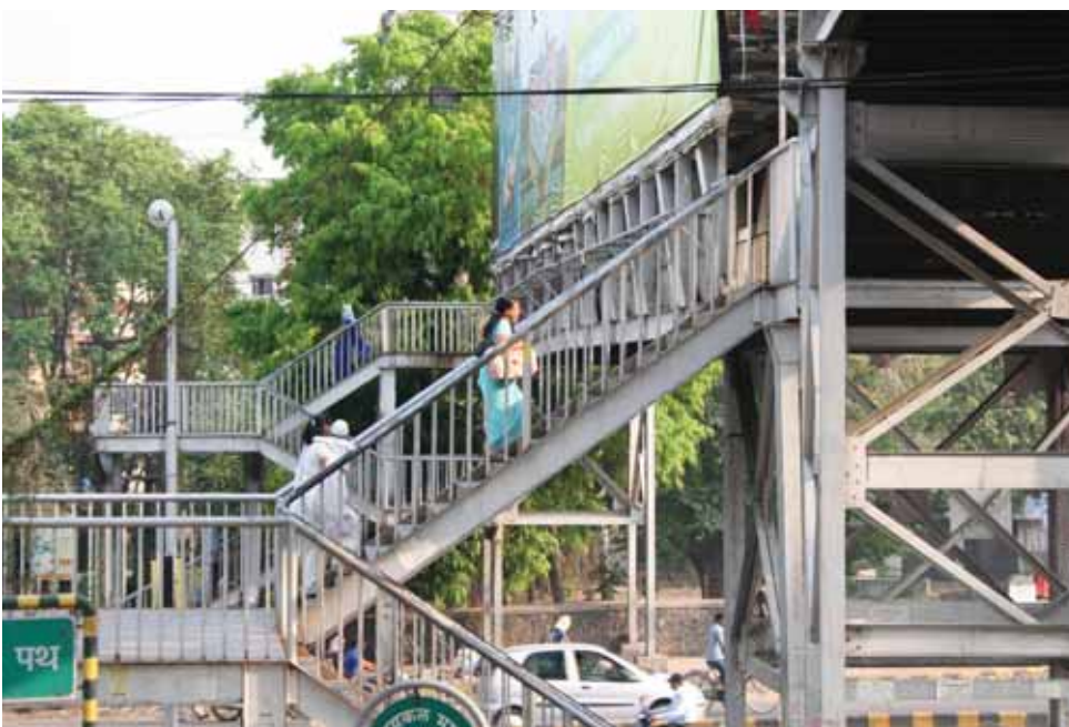
FOB on Satara Road is particularly difficult for women carrying infants
